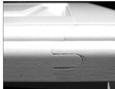
Example of end joint separation
