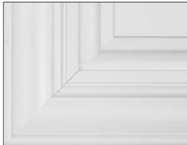
Example of front joint separation
