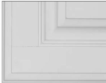
Example of front joint separation
