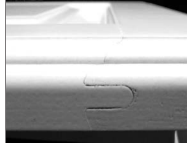
Example of end joint separation
