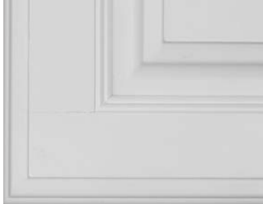
Example of front joint separation
