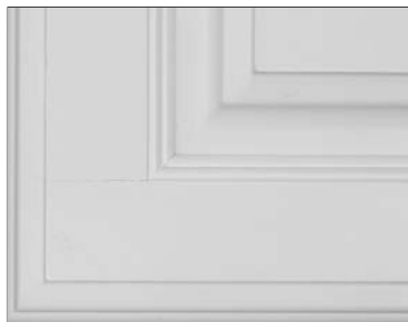
Example of front joint separation
