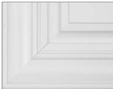
Example of front joint separation
