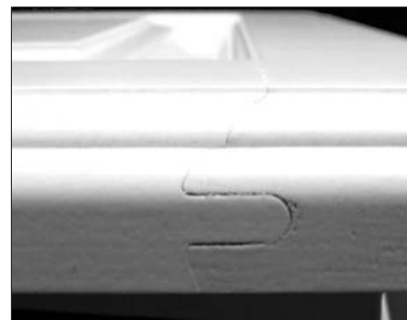
Example of end joint separation
