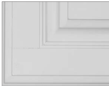
Example of front joint separation
