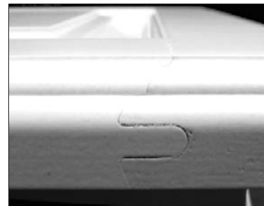
Example of end joint separation
