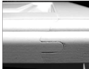
Example of end joint separation
