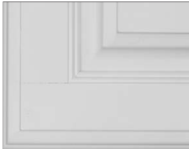
Example of front joint separation
