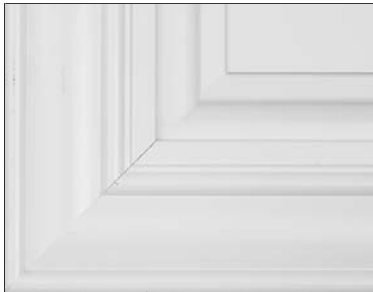
Example of front joint separation
