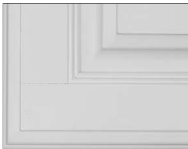
Example of front joint separation
